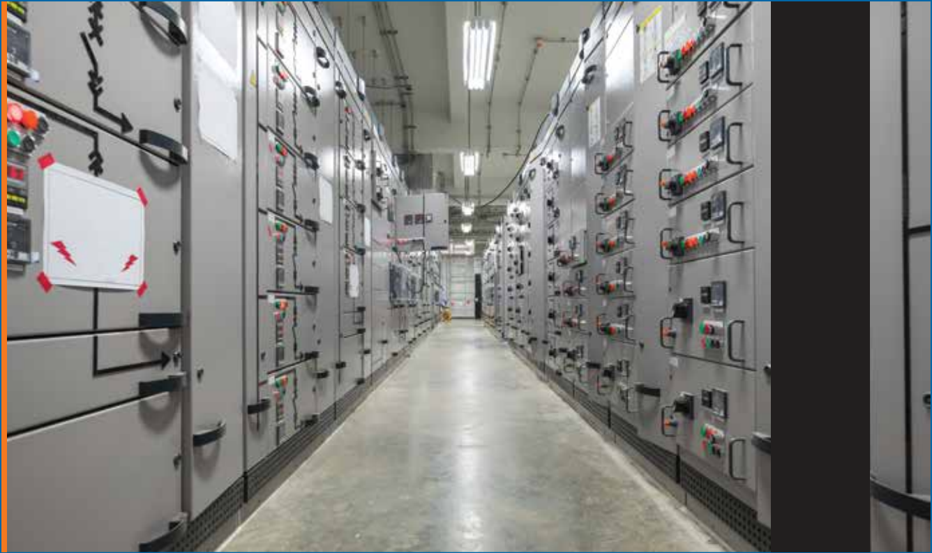
Switchgear Rooms: Illumination Level: 200lux
